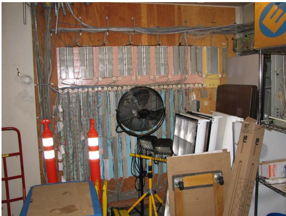
Items stored right in front of the termination field in Building 2471 – IDF 1.1. Items should be removed or displaced to the side for easy access and work space clearances.
