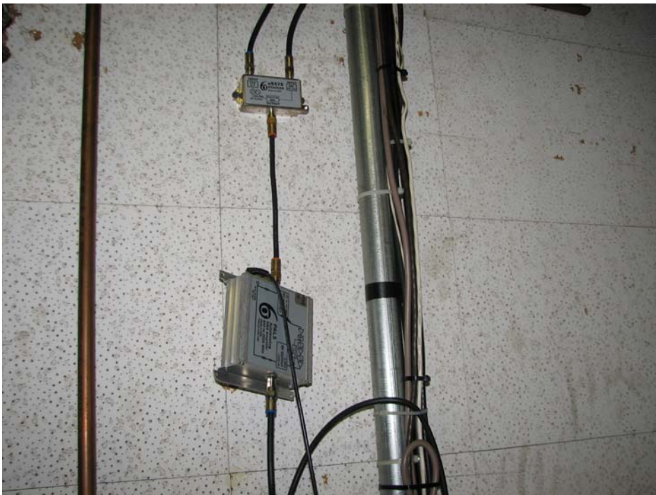
Coax cable located inside the Mechanical Room in Building 2465 – second floor. These cables pass through a conduit and into the ceiling space of the first floor. The final destination is unknown but is expected to be in suites.
