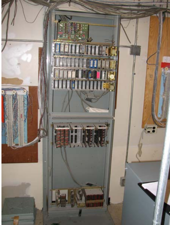
Equipment rack in Building 2483 – IDF 1.1 that is expected to be abandoned and not in use.
