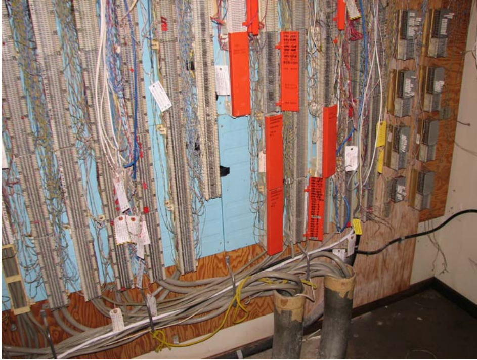
Some additional termination points for the IDF feeders in the MPOE.
