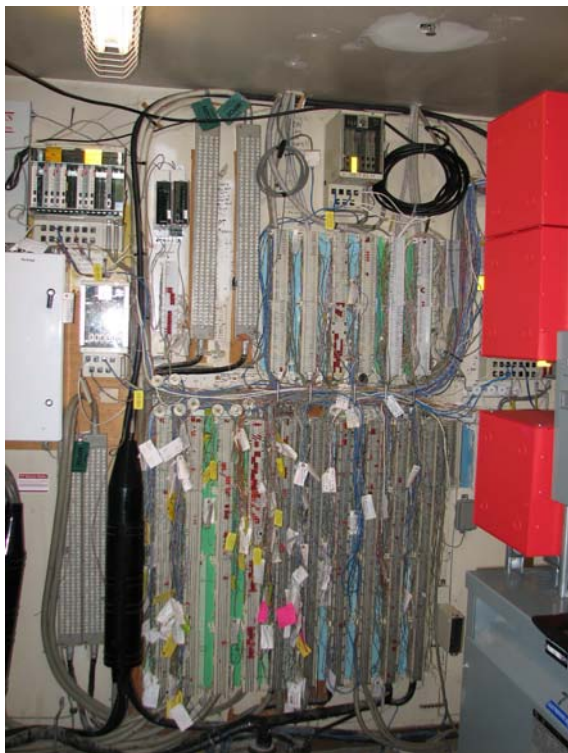
This is the entry point from the “street” (LEC) for the copper Telco Facilities, fused protection field and termination point. The blue field is for the IDF feeders.
