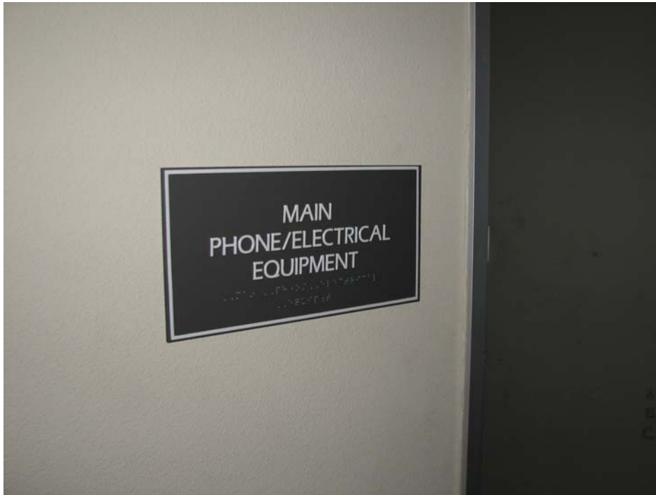
The MPOE location in Building 2465 – first floor. The MPOE has an interior access only.
